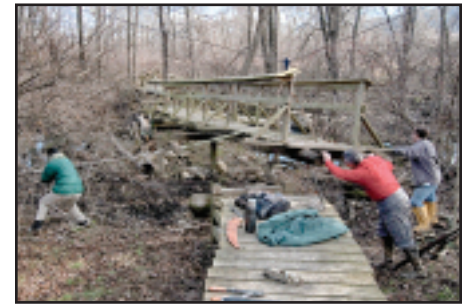
A bridge is replaced on the Appalachian Trail along the Pochuck Canal.
